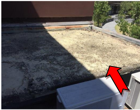
7. Surgery, exterior, rooftop, lower elevated area, throughout - asbestos-containing bituminous material.
