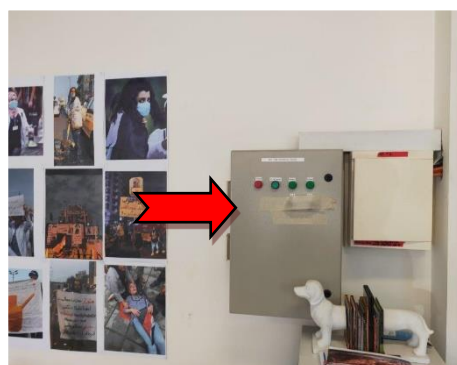
2. Studio 52, interior, south wall, air handling control panel, switchboard – assumed asbestos-containing bituminous backing board.
