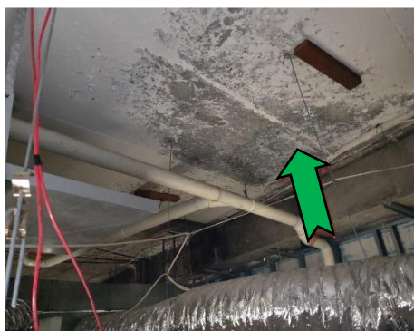
4. Studio 52, interior, ceiling space, throughout – non-lead paint containing grey upper coloured paint system debris.
