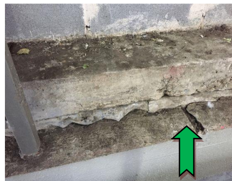
11. Crunch Fitness Car Park, interior, level B, northern elevation adjacent AC cage stairs, dust – non-lead containing dust.
