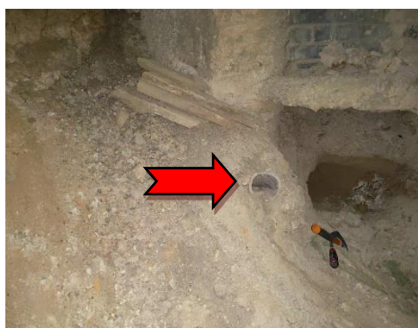
5. Crunch Fitness, interior, subfloor adjacent loading dock, pipe work, throughout – asbestos containing moulded fibre cement.
