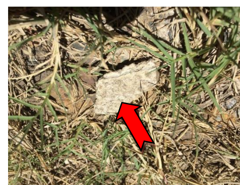
12. Grassed area between Crunch Fitness Car Park and Just Sports tenancy, centre, on ground – asbestos-containing fibre cement sheet debris.
