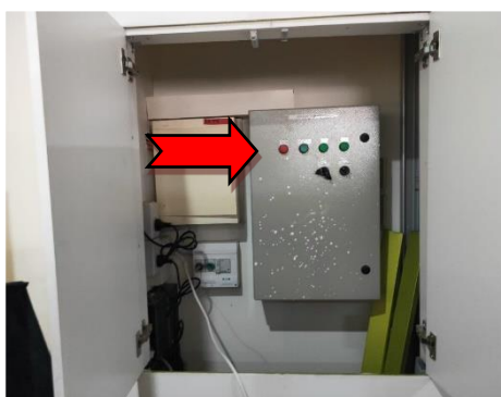
1. The Rising Collective, south corner, switchboard – assumed asbestos-containing bituminous backing board.
